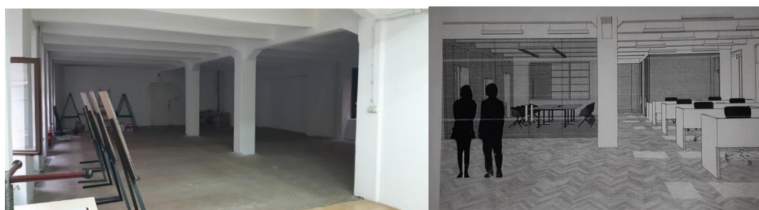
The new Reading room under construction and its planned appearance after completion of the works
