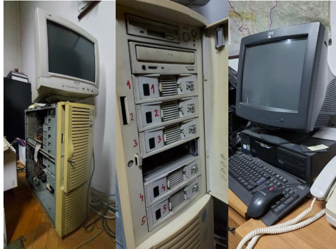
Photo 5,6 and 7 – Outdated IT equipment can easily lead to permanent data loss
